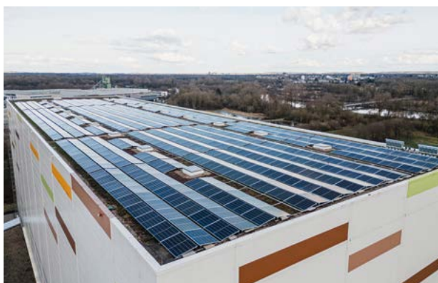
Photovoltaic panels on the high-bay warehouse
